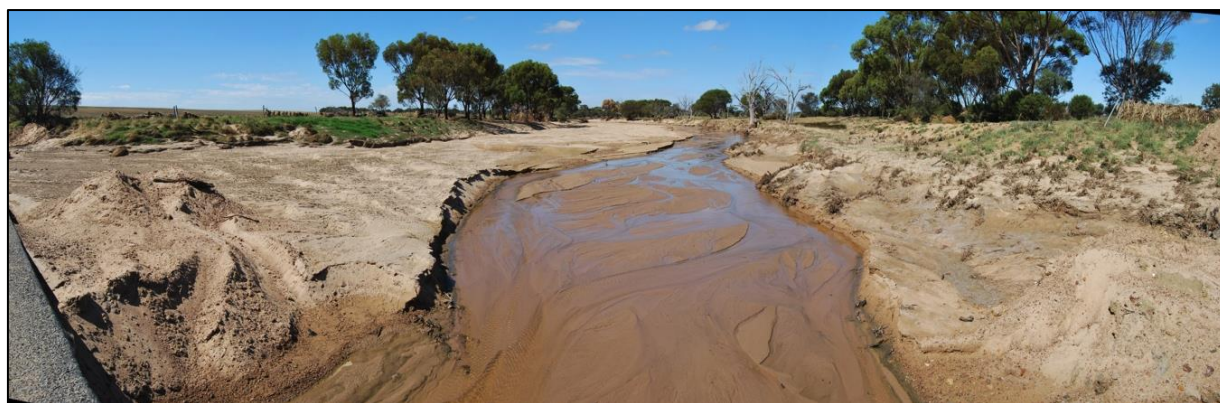
Jackitup Creek at Formby South Road crossing in March 2017 - looking upstream.
