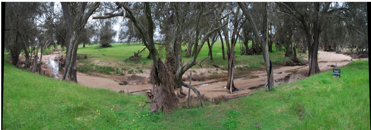
Willemenup Creek - second confluence. The channel is choked with sediment and extensive deposition and unprotected banks appear to extend upstream at least as far as Camballup Road (1.2 Km)
