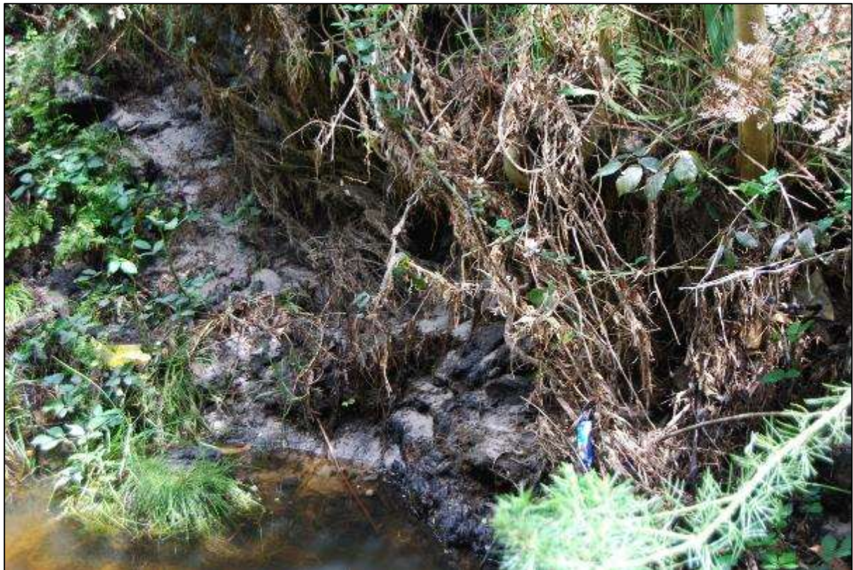
Figure 18: The water's edge (toe of the bank) of Yakamia Creek where the banks are steep and collapsing (Section D2.4)
