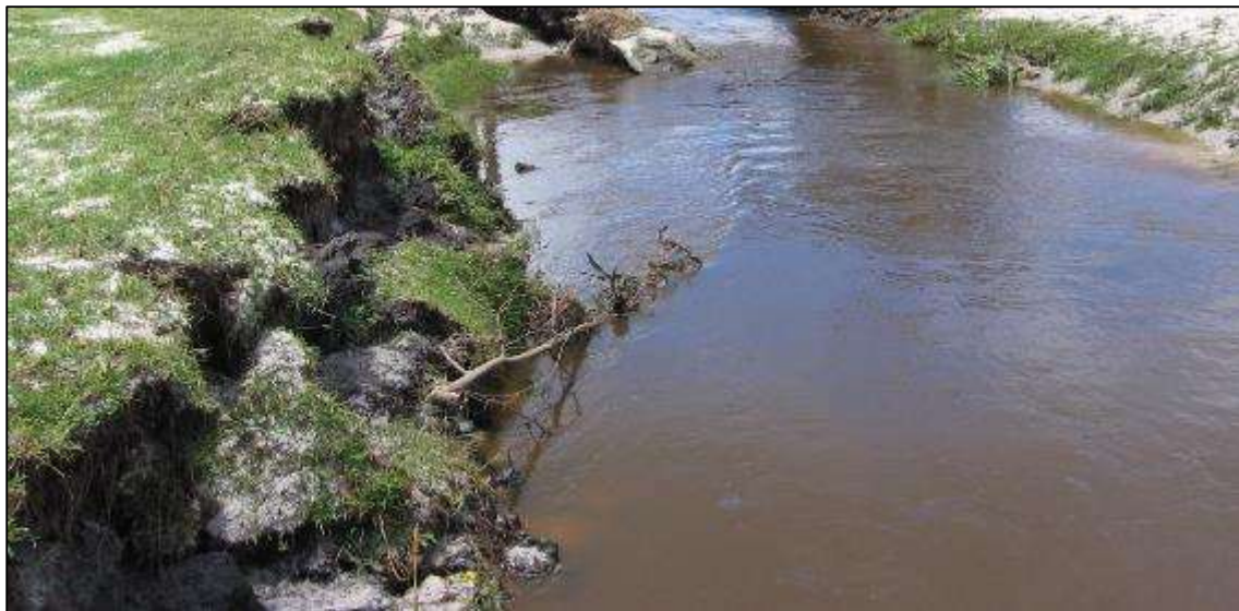
Figure 17: Bank collapse under kikuyu grass after the 2008 flood, Photo courtesy of Wilhelm Ficko
