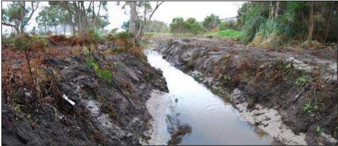
Figure 5: Aggressive channel excavation along section C3 below North Road tends to promote weed growth and encourage bank erosion.
